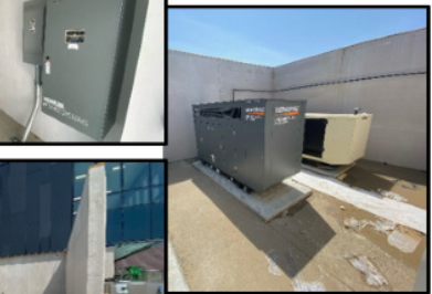
Ames High School (new generator & tank location)
