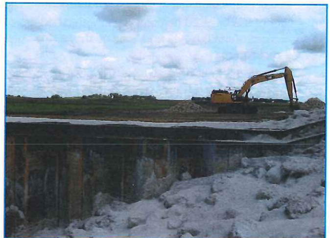
Construction underway at a CREP wetland located in the Boone River watershed
