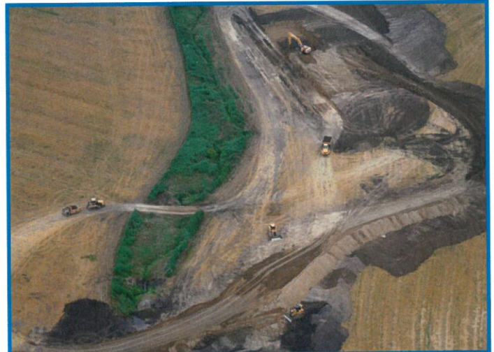
Construction of targeted wetland restoration in Wright County photo courtesy of Bruce Voigts
