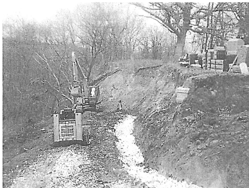
Dec. 2011: Work to build a retaining wall at Oak Grove Cemetery in Lehigh.
