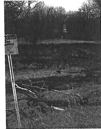
This stream has downcut enough that a once buried gas pipeline was exposed and then severed by a falling tree in Nebraska.
