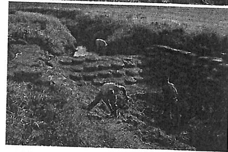
Top: Scrap tire project after initial construction. Bottom: Loose cement removed and the scrap tires have been filled and covered with flowable concrete grout.
