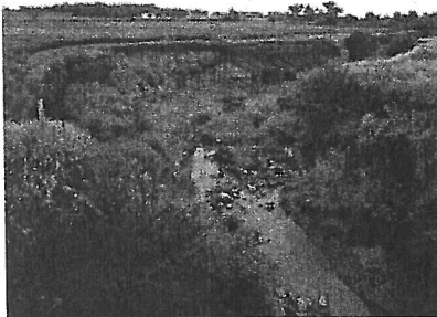
Degradation on this stream has caused the near-vertical actively-eroding streambanks in Nebraska.
