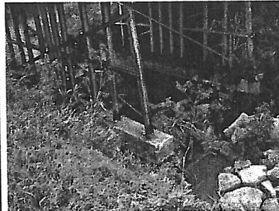
This stream has downcut enough that once buried footings on a major state highway bridge in Nebraska have been exposed, endangering the bridge.
