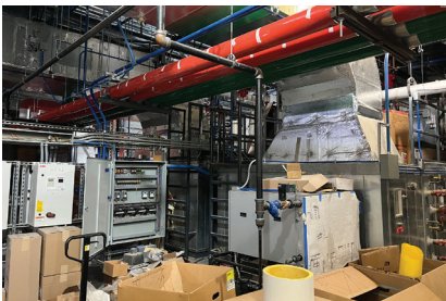
◀ left: mechanical room
