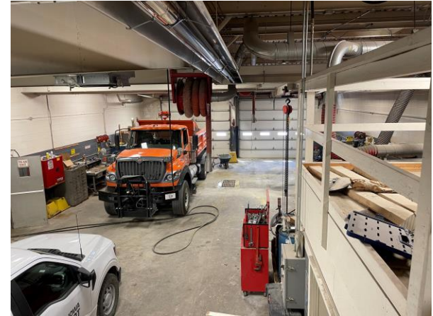
Vehicle height and length operational clearance insufficient for new trucks and attachments.
