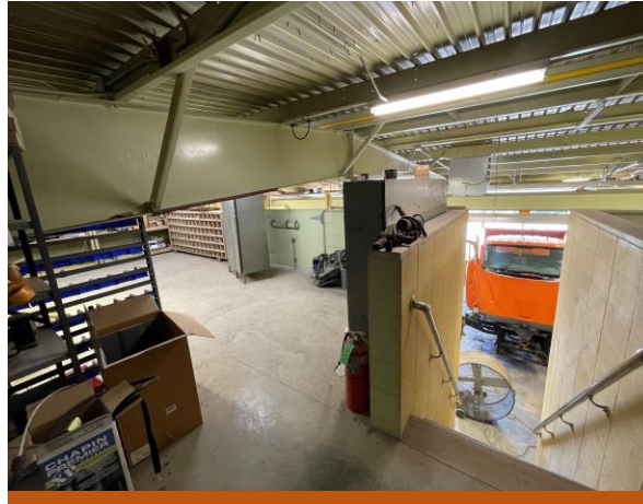
Insufficient space at front and back vehicle in mechanic's stall. Second floor store room does not meet ADA or Building Code.
