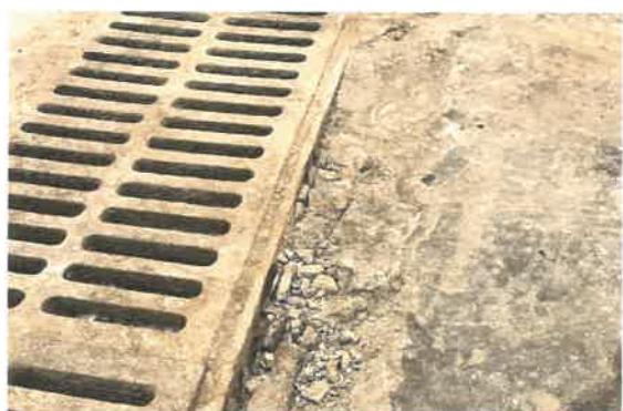
Older style trench drains create concrete floor and sewer maintenance problems.
