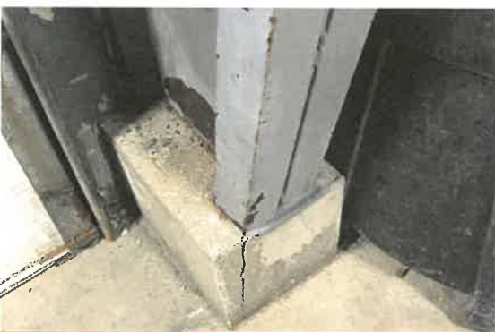
Structural columns and foundations are beginning to deteriorate.
