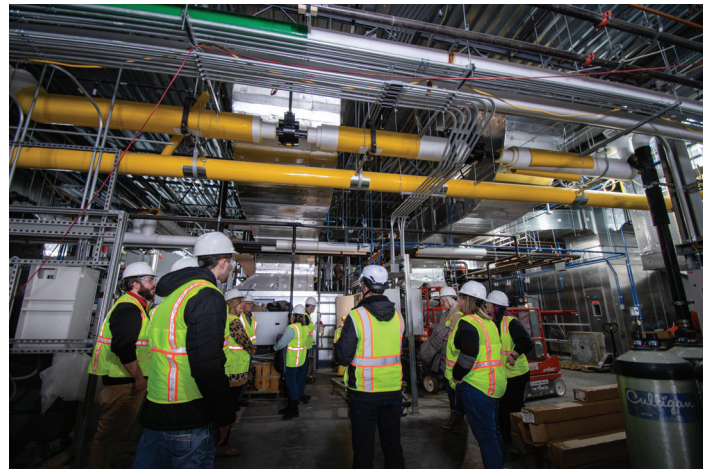
▲ above: one of several mechanical rooms
