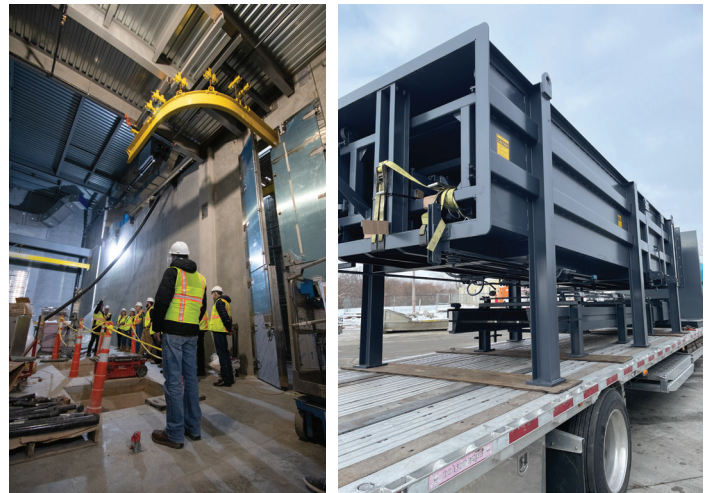
▲ above: the incinerator room and a portion of the incinerator on a transportation trailer
