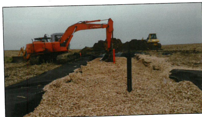
Bioreactor installed in Keokuk County
