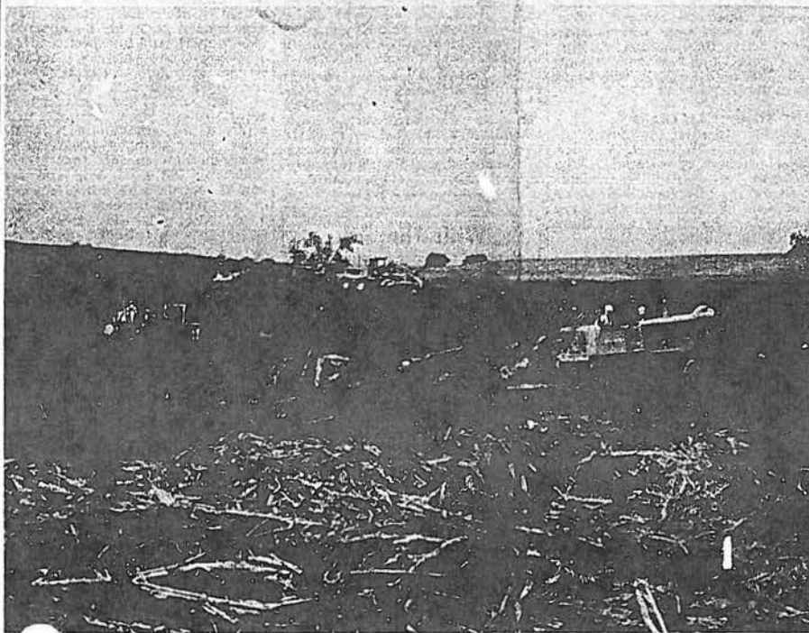
Work on a large structure was one of the features of the Conservation Field Day last week on the Turner and Hogan farms north of Corning. Photo above shows contractors at work carrying and pushing dirt to the top of the structure which measured 350 feet long and 12 feet wide at the top.—Free Press photo by Phil Gauthier.
