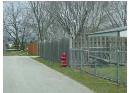
New fire hydrant in the distribution system
