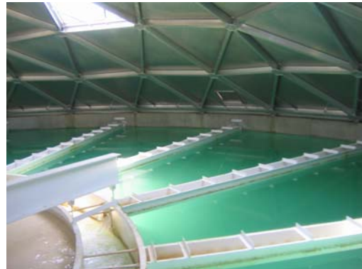
Lime softening basin and weir
