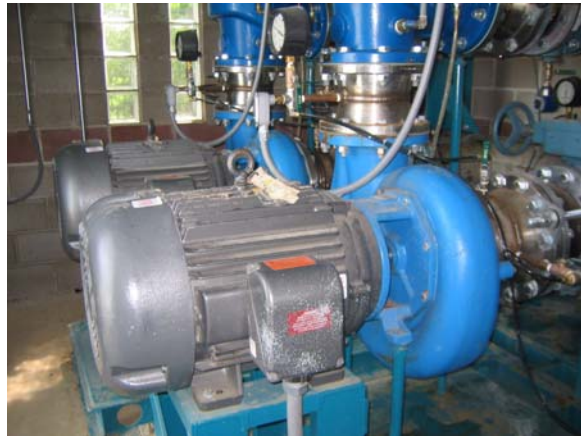
Booster pump station
