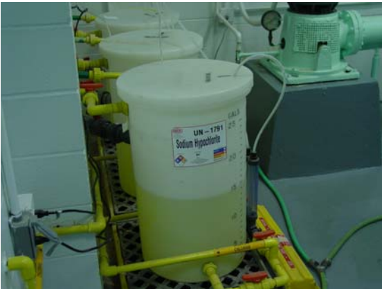
Chlorine solution for disinfection
