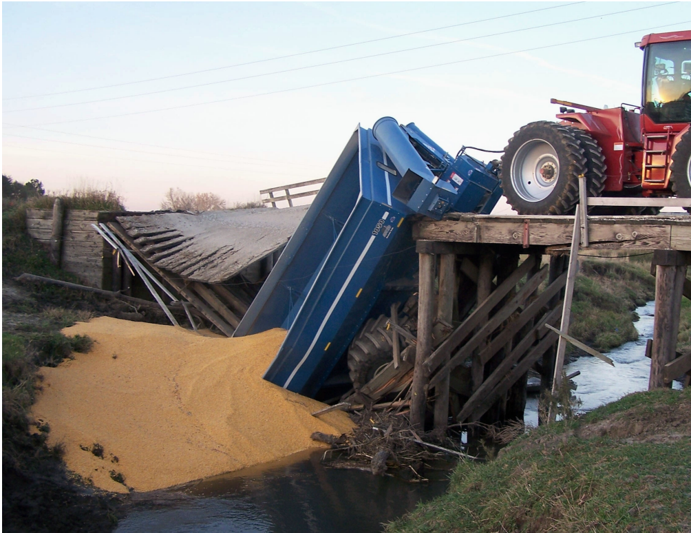
Collapsed bridge on Eagle Place Road in Audubon County
