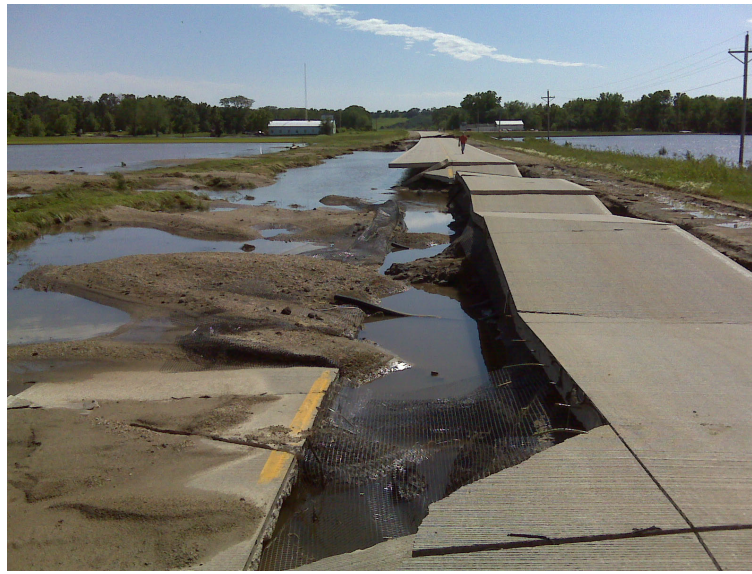
Flood damage to Iowa 1 in Linn County
