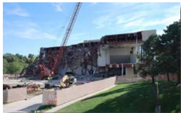
Recovery work on Hancher Auditorium at the University of Iowa, which sustained severe damage during flooding in 2008.
