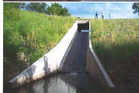
Top: 4 foot high sheet pile weir with a 1:20 gouted riprap slope in Crawford County. Bottom: RCB flume with 25 feet of fall in Fremont County.
