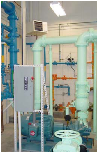
Pump & pipe gallery
