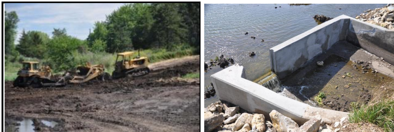
Sediment removal and new box culvert at Lake Anita east silt pond in 2013.
