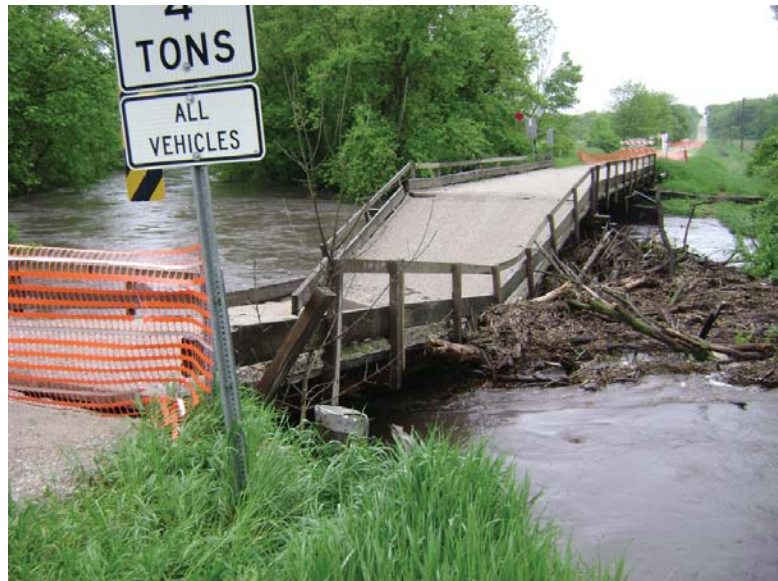
Damage to a bridge in rural Story County during the May-June 2013 flooding.
