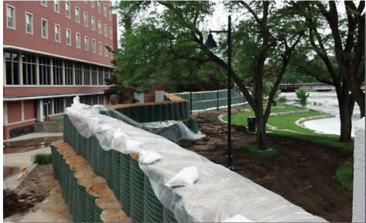
Flood barriers erected at the Memorial Union on the University of Iowa campus in May 2013.
