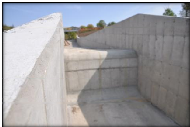
Prairie Rose Lake spillway was modified to add a 9-foot drop to prevent undesirable fish from entering the lake from below.
