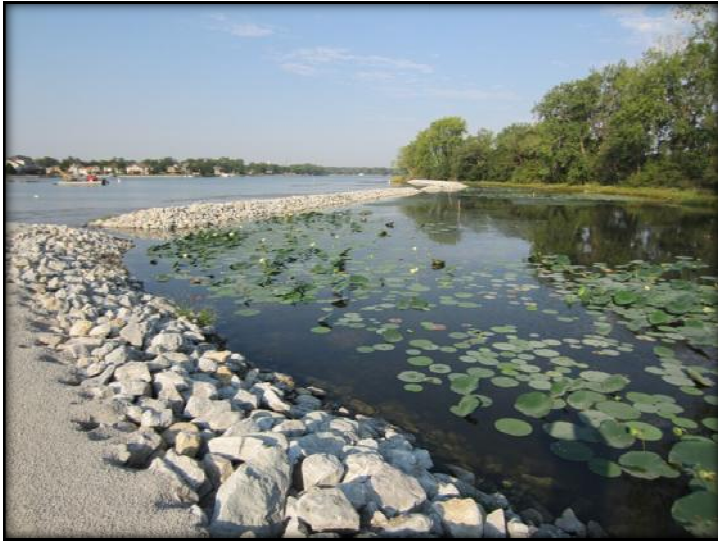
Contractors completed shoreline armoring, off-shore breakwaters and a new storm water basin on the north side of the lake in 2012
