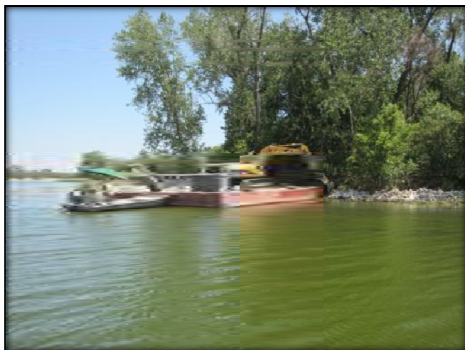
Tetra Tech engineered wetland restoration and shoreline protection measures for 2012 spring/summer construction. Image shows shoreline armoring at Carter Lake from a barge in 2012.
