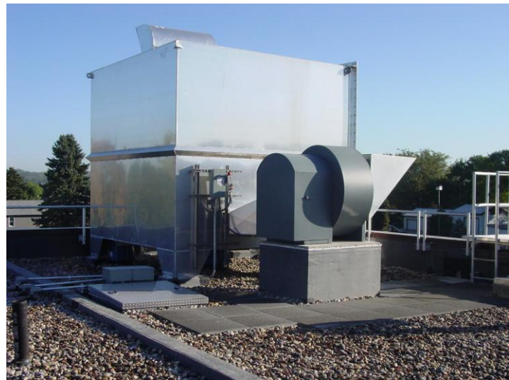
Aerator installed as part of a DWSRF project that was completed in 2011
