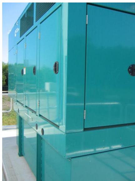
Generator for Emergency Power Generation installed as part of a DWSRF project completed in 2011
