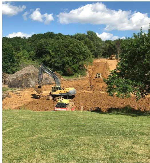
Construction at one of the watershed ponds constructed in the part as a part of the restoration efforts.
