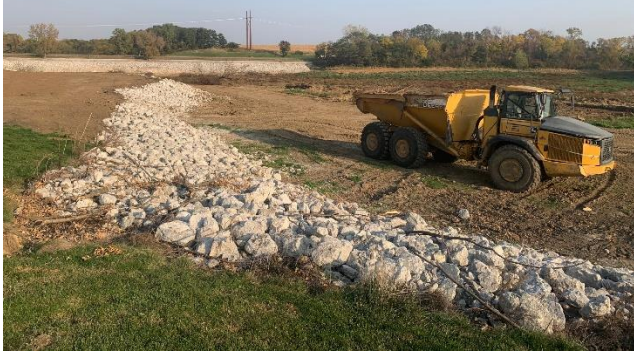
Shoreline stabilization along the banks of Lake of the Hills. Over 1000 feet of shoreline are being armored as a part of this project.
