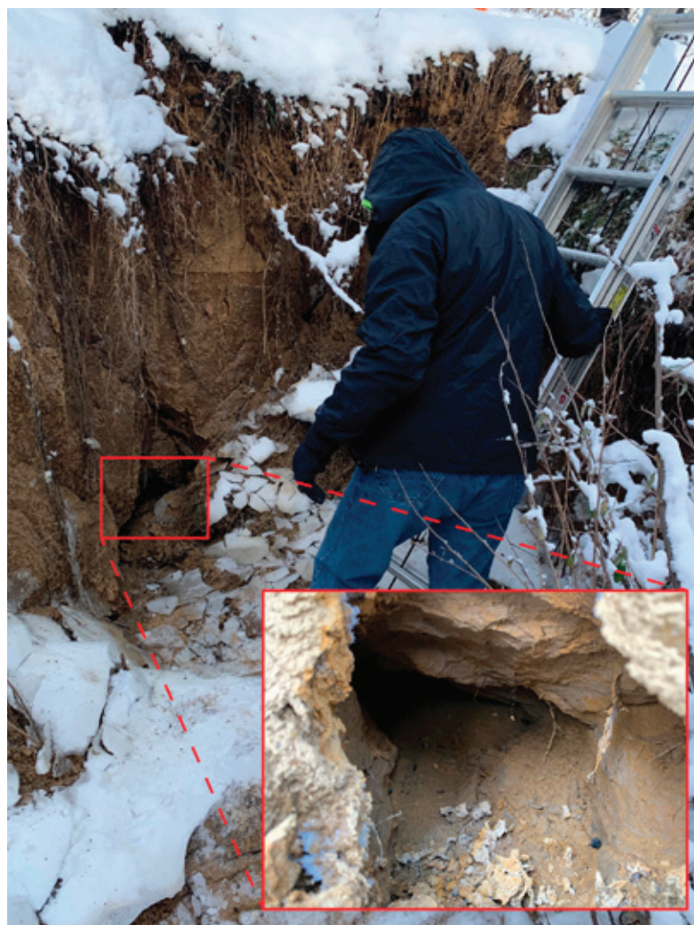
FIGURE 1. Visual inspection of the sinkhole revealed the point where water (and sediment) likely escaped into the subsurface.
