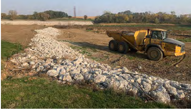
Shoreline stabilization along the banks of Lake of the Hills. Over 1000 feet of shoreline are being armored as a part of this project.
