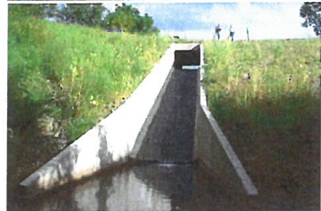
Top: 4 foot high sheet pile weir with a 1:20 grouted riprap slope in Crawford County. Bottom: RCB flume with 25 feet of fall in Fremont County.
