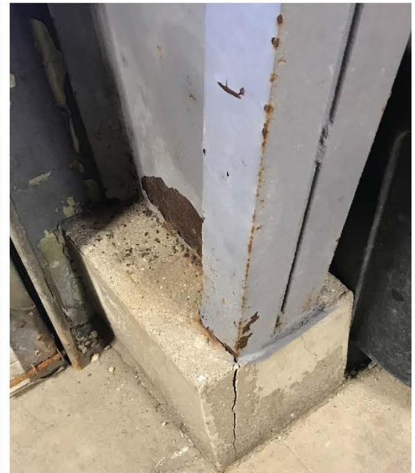
Structural columns & foundations are deteriorating.
