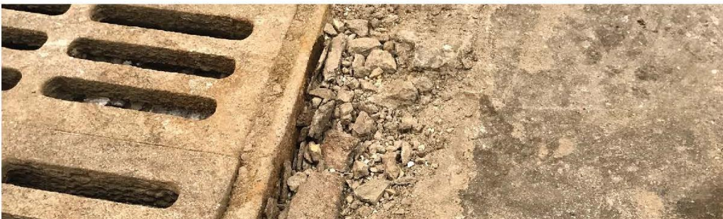
Older style trench drains create concrete floor and sewer maintenance problems.
