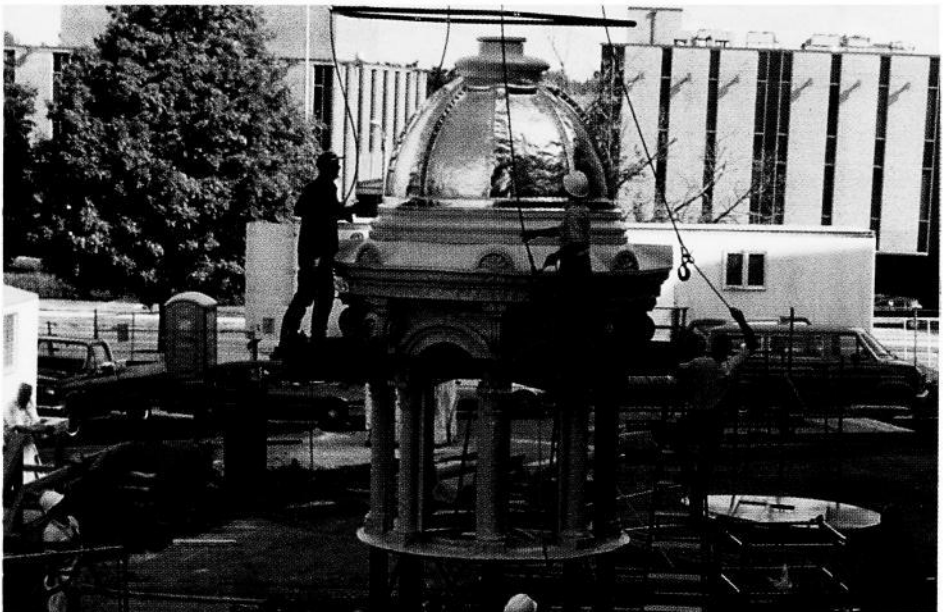
Workers prepare to raise one of the small domes to the top of the Iowa State Capitol after restoring it to its original splendor.
