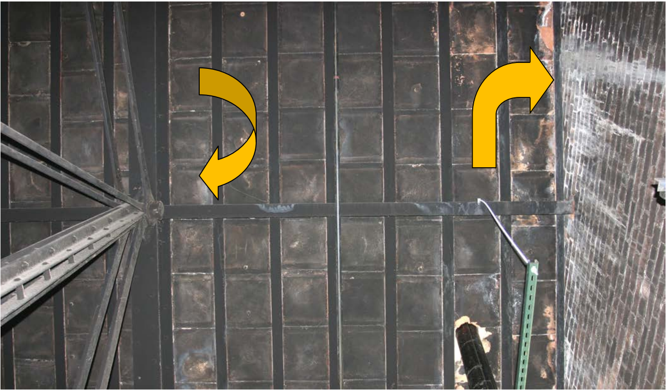
Soot and water stains remain on the walls and ceilings in the north attic more than a century after the fire.
