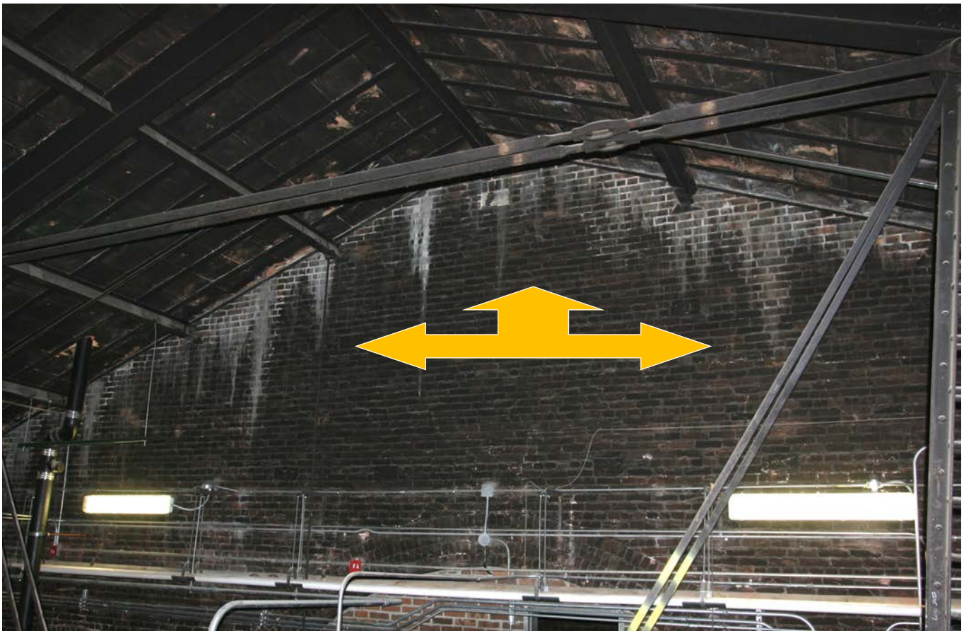
Soot covers the north wall and ceiling of the attic above the House Chamber. Water used to fight the fire streaked areas of the brick wall.
